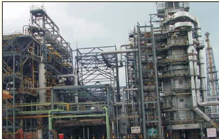
Diesel Hydrotreater Project in Visakha Refinery
